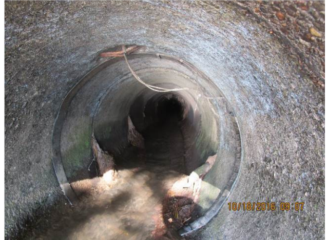
Picture 8 – Clear Water Pond, root intrusion at end of discharge pipe
