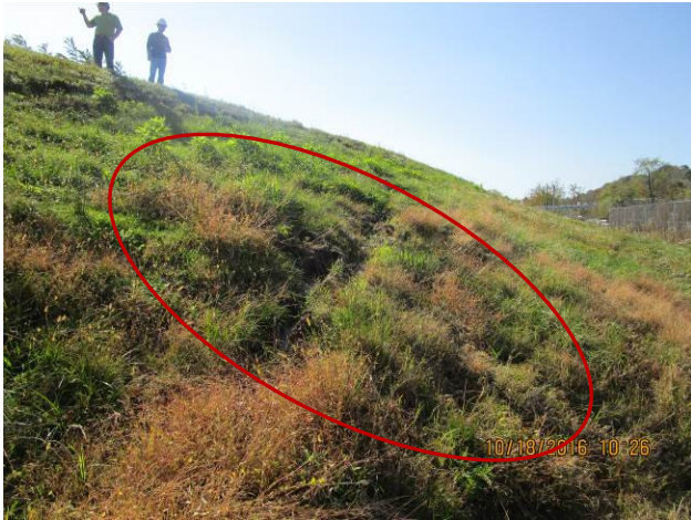
Picture 18 – South Fly Ash Pond, wet area at south-west dike
