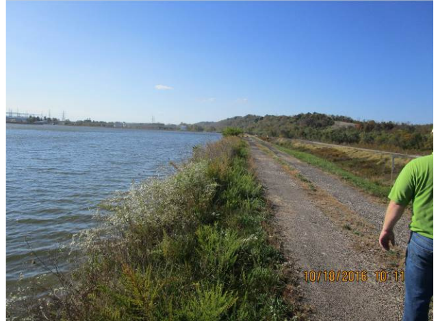
Picture 11 – South Fly Ash Pond, excessive vegetation along inboard slope
