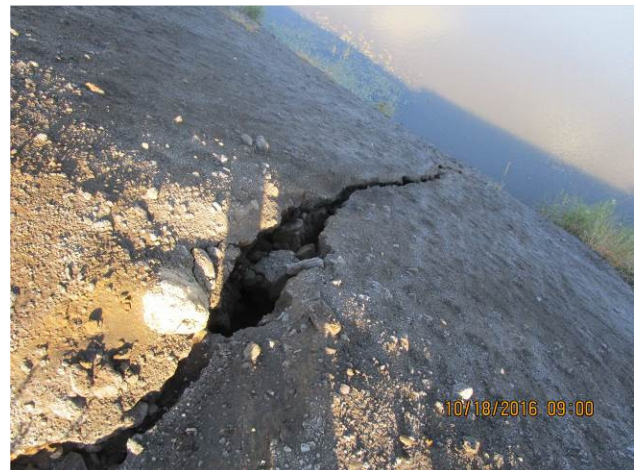
Picture 6 – Boiler Slag Pond, erosion on inboard slope
