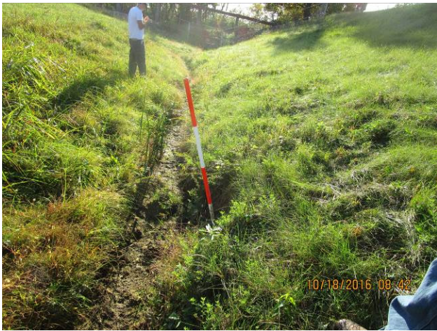
Picture 3 – Boiler Slag Pond, abandoned appurtenance at north toe
