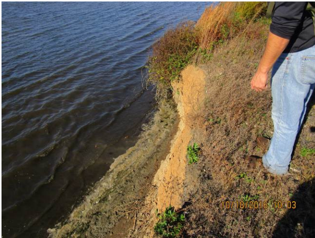
Picture 12 – South Fly Ash Pond, wave erosion at north dike inboard slope
