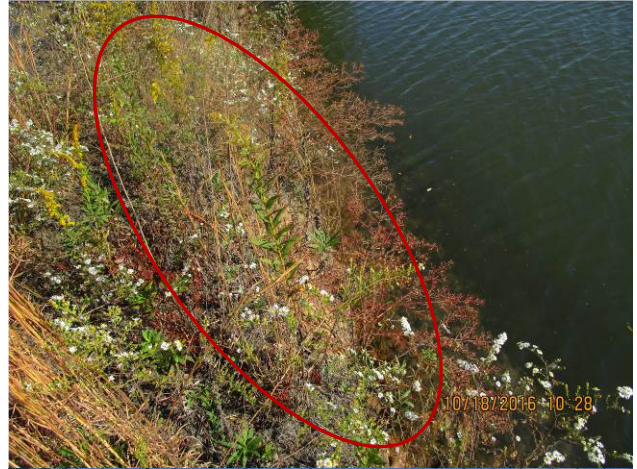
Picture 17 – South Fly Ash Pond, wave erosion at west dike inboard slope
