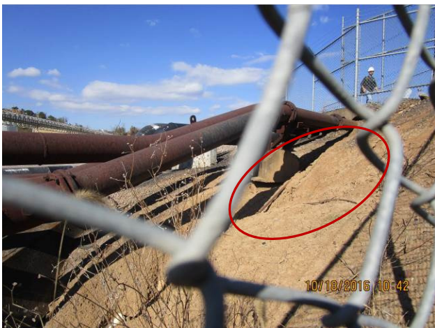
Picture 20 – South Fly Ash Pond, erosion at south dike outboard slope near the sluice line
