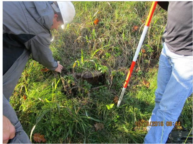
Picture 4 – Boiler Slag Pond, abandoned appurtenance at north toe
