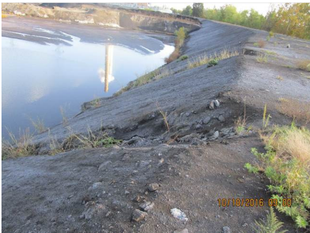
Picture 5 – Boiler Slag Pond, erosion on inboard slope
