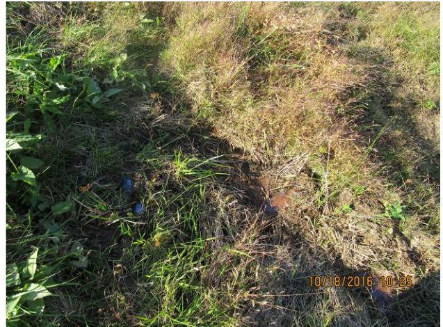
Picture 19 – South Fly Ash Pond, wet area at south-west dike
