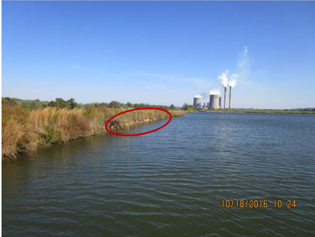
Picture 16 – South Fly Ash Pond, wave erosion at west dike inboard slope
